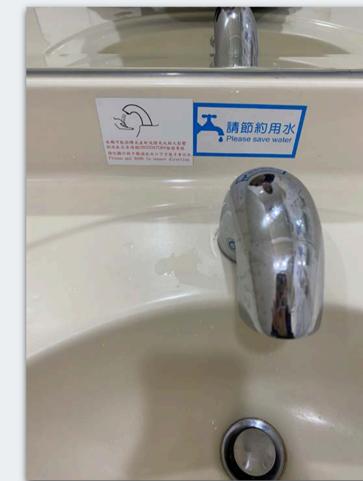
Installing auto-sensing faucets to avoid contact infection
