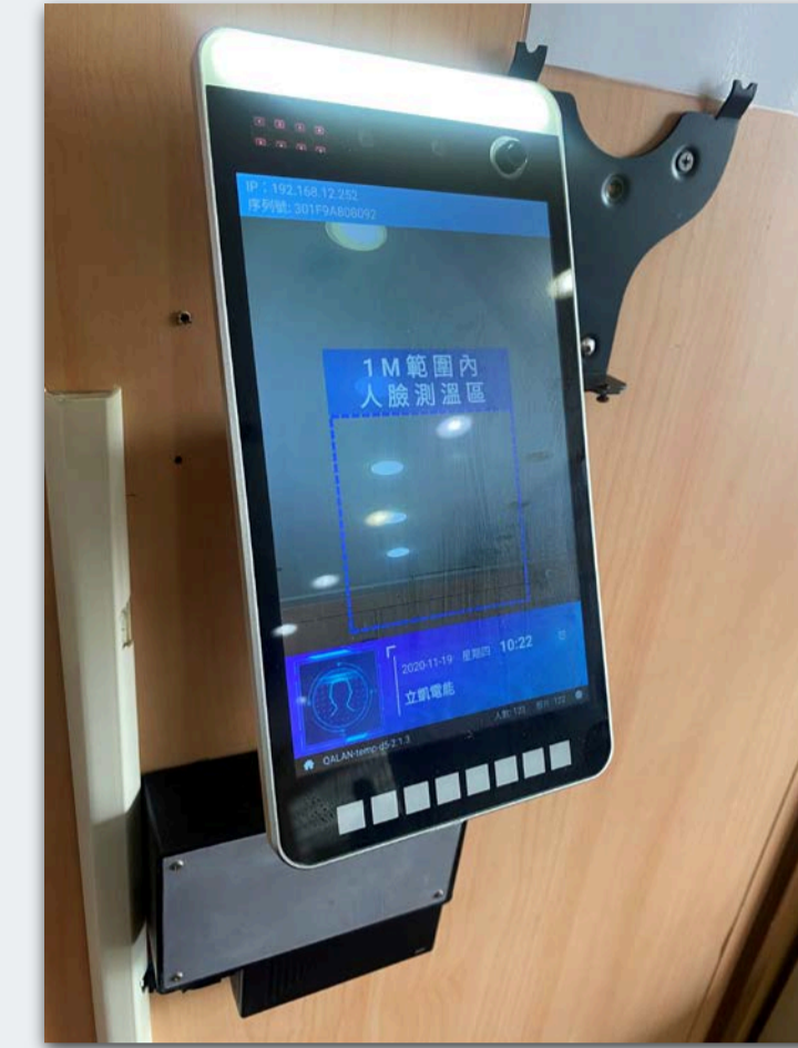
Measuring body temperature at clock-in and clock-out to control personnel access
