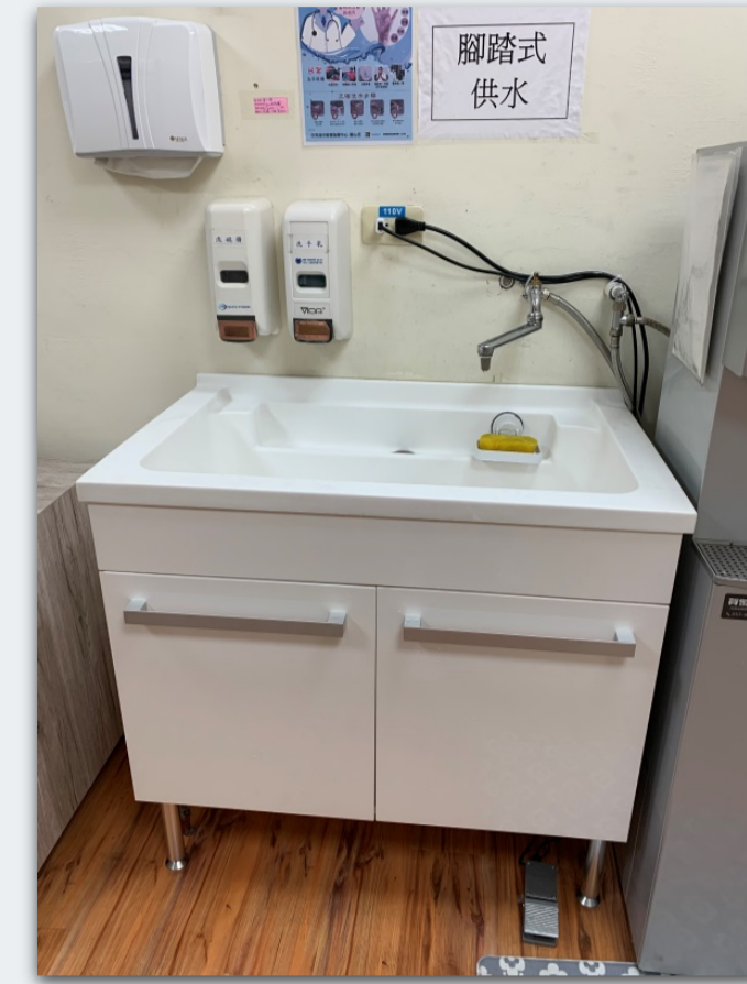
Replaced with pedal faucet and sensor faucet
